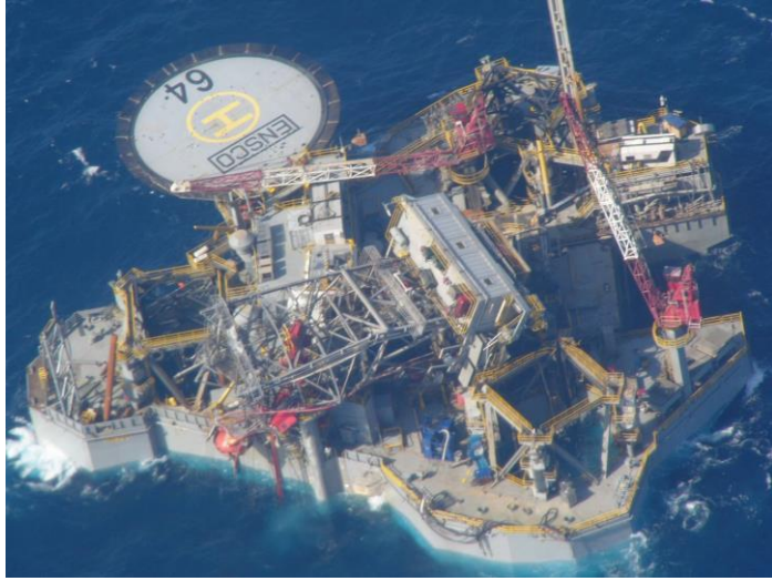
Post Hurricane Ivan, ENSCO platform off the Louisiana Coast
